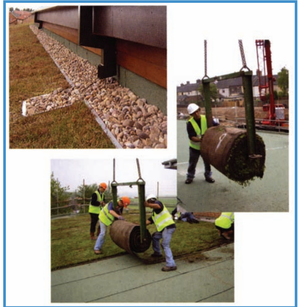
“delivery and installation of sedum rolls and detail of abutment” (Courtesy of Bauder Ltd)
